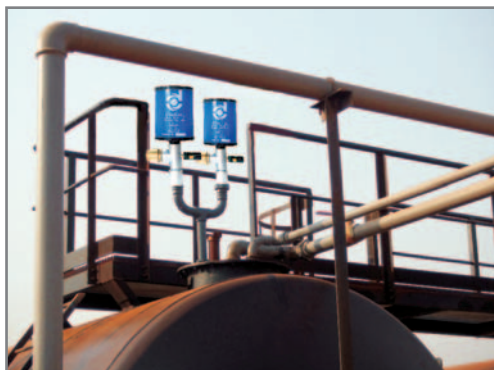
T.R.A.P. Breather installation on a bulk tank
